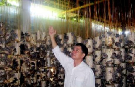
Dr. Ai checking internal lines of the automatic water cooling system operational in a mushroom growing house.
