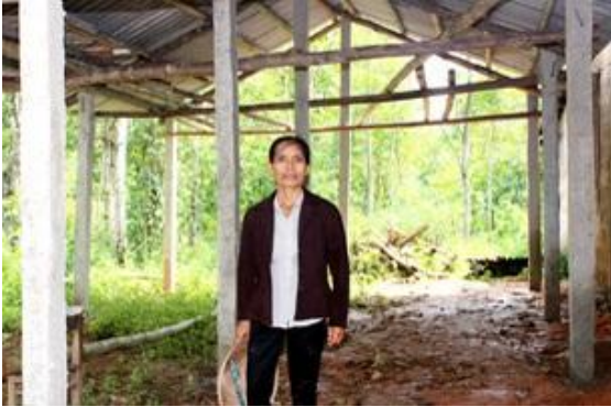
Construction on Ms. Muon's new rainproof mushroom growing house, built with support from the MWM, is nearly finished. She will soon be growing Lingzhi mushrooms for the first time, expected to bring her a very good income.
