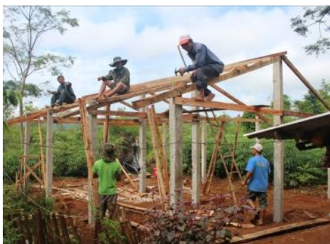
50 farmers received new grow houses to grow Linh Chi mushrooms. Here construction workers are putting the roof on a grow house.
