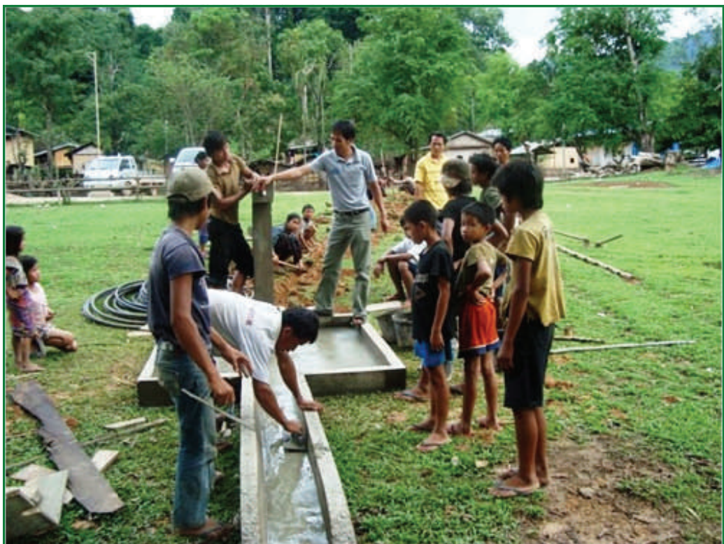
Completing the construction of the water pump in the school ground for the gravity-fed water system in Thongkong Village
